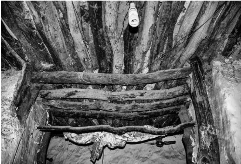
Fig. 41 Banda Nkwanta, detail of the ceiling of the prayer hall (photo Denis Genequand).
