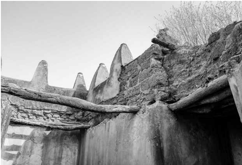
Fig. 39 Wa, Dondoli mosque, different mud-brick masonry types in the qibla wall and the northern wall (photo Denis Genequand)
